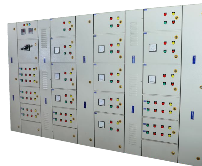
Motor Control Center Panel
